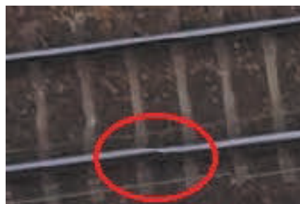
Figure 2. Discontinuité du rail
